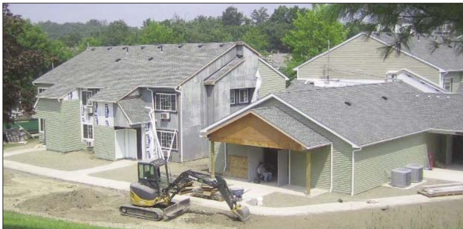
Community Services Programs Inc. completed top-to-bottom renovations at Green Meadows Apartments that transformed and preserved 36 units of affordable housing in Chester, New York.
