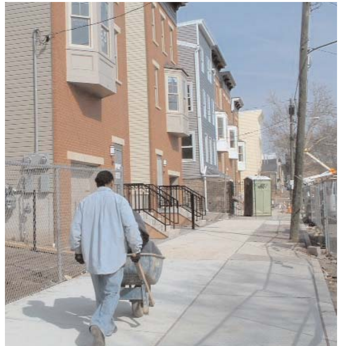
Workers handle final phase of construction at La Casa's new homes in Newark. First new residents will arrive in early May.
